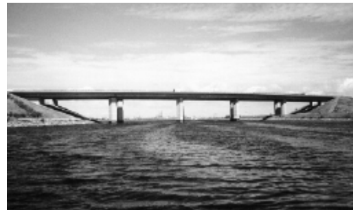
Figure 9 Example b) : Typical Danish coastal RC columns which may require repair after 20-40 years.
