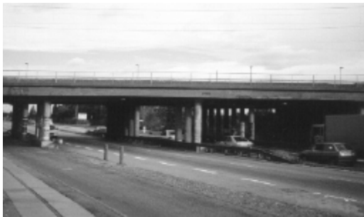
Figure 8 Example a) : Typical highway RC columns requiring repair or replacement after 20-30 years.
